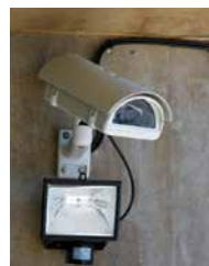
Exterior Security Lighting
